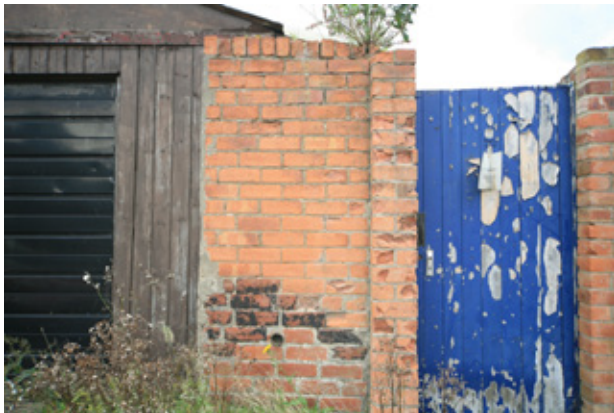
Figure 8.10.19; Some parts of the character area are in a poor condition
