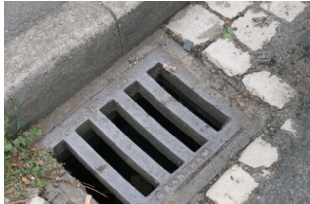
Figure 8.1.50; Retention of stone gully setts and traditional locally made street fittings is important to maintaining the character of the town centre
