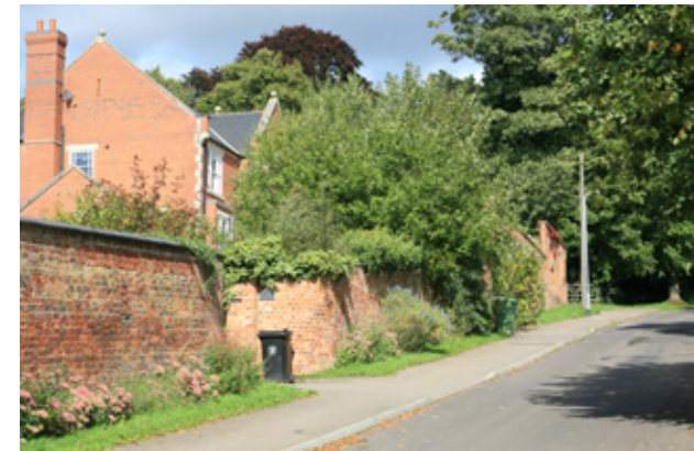
Figure 8.7.12; Remnant survival of heritage assets (brick boundary wall to grounds of St Vincent's (CA08a)
