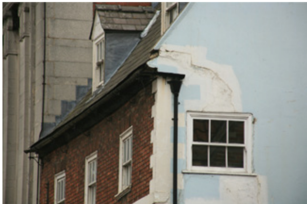
Figure 8.1.46 and Figure 8.1.47; Some buildings within the town centre are showing signs of neglect. Many upper floors are underused or vacant leading to lack of investment and maintenance.
