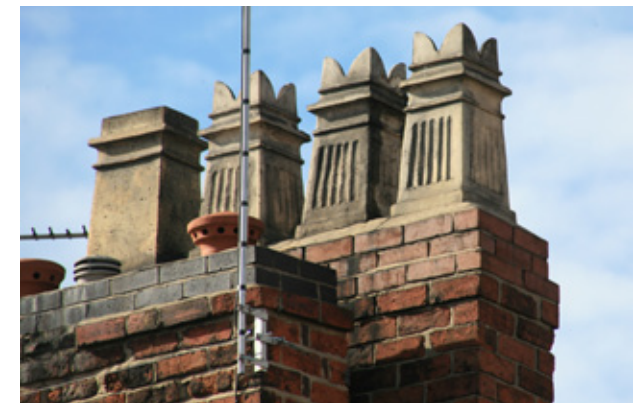
Figure 8.3.19; Decorative clay pots to chimneys
